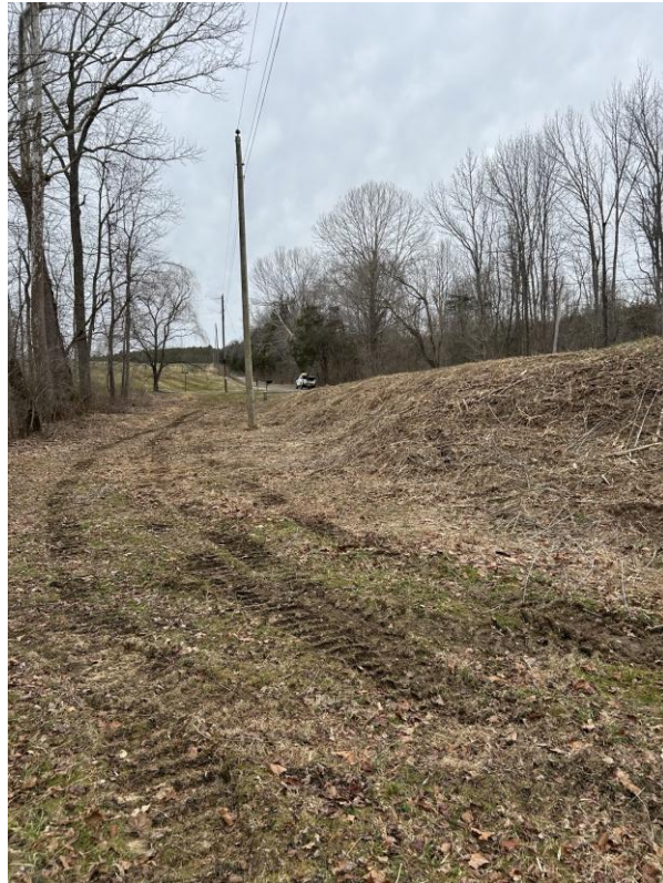
Figure 13. Detail view of vegetative clearing on Lecky Property (Hard Bargain), looking west
